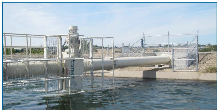
Fig. 6. This ultra-low-head pilot project with limited civil works (no dam, penstock, drop, or weir required) was deployed at the Bureau of Reclamation Roza Canal on the Yakima Project in Washington. The design spans the canal, which prevents contact with the canal lining and limits waterway interactions.
