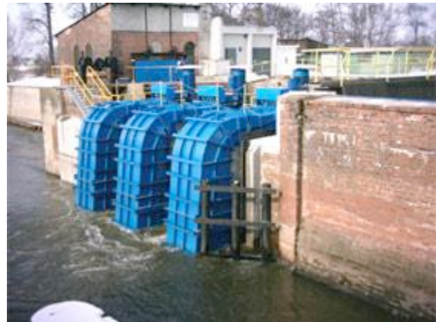
Fig. 2. This siphon turbine was installed on an existing weir in southern Poland in 2006. The same company is constructing the Head of the U hydropower project in Idaho using this technology.
