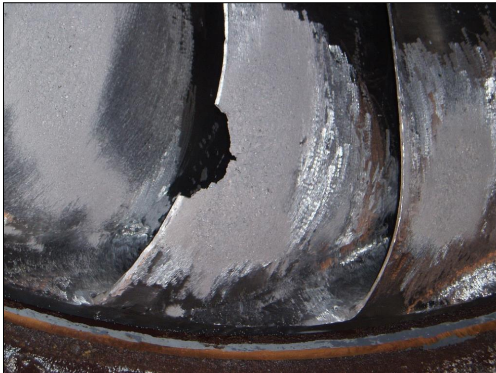
Figure 2.4 Cavitation Damage on a Turbine's Runner Blade at Fremont Canyon Power Plant in Wyoming (USBR facility)
